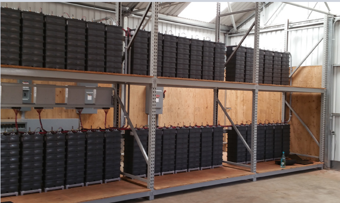
Forty Aquion battery stacks are used to power a 25-kilowatt installation at Mari's Garden, a nursery in Millani, Hawaii. The business's heavy power demand – combined with high Hawaiian electricity costs – made combining a solar PV array with Aquion batteries a smart financial decision. (Photo courtesy of Aquion)
